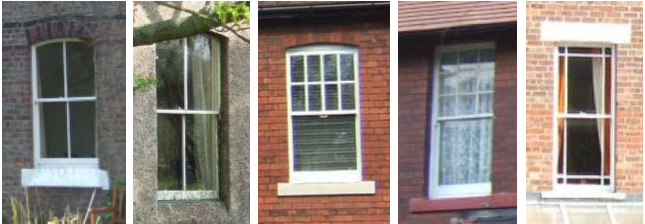
Victorian and Edwardian sliding sash windows, some with glazing bars only in the upper sash as decoration
