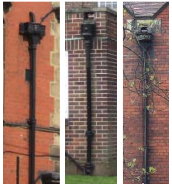
Iron hoppers & drainpipes: frmr institute, Health Cntr, H'n Vs
